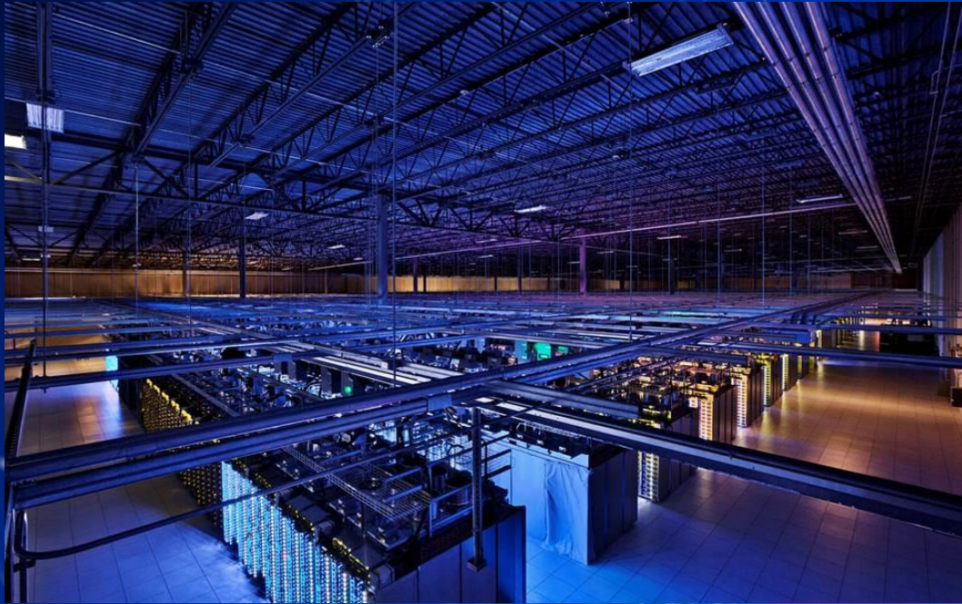
Google data centre – Iowa, USA
